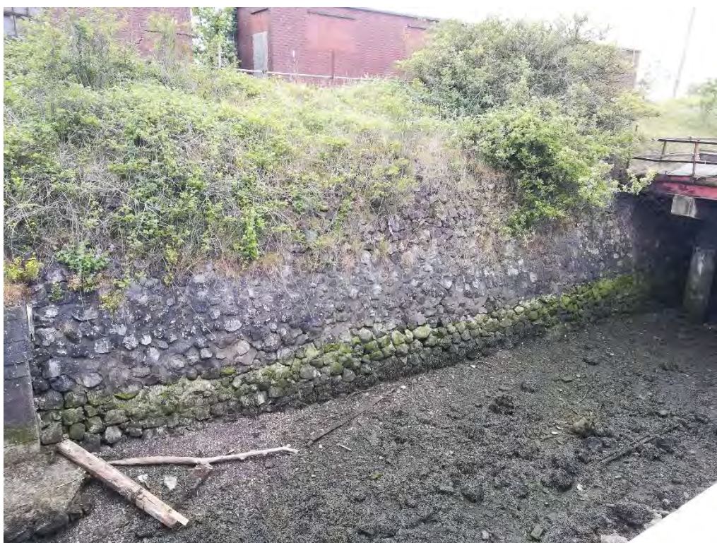
Plate 28.1 Intertidal area to be lost as a result of excavation to create the berth pocket
